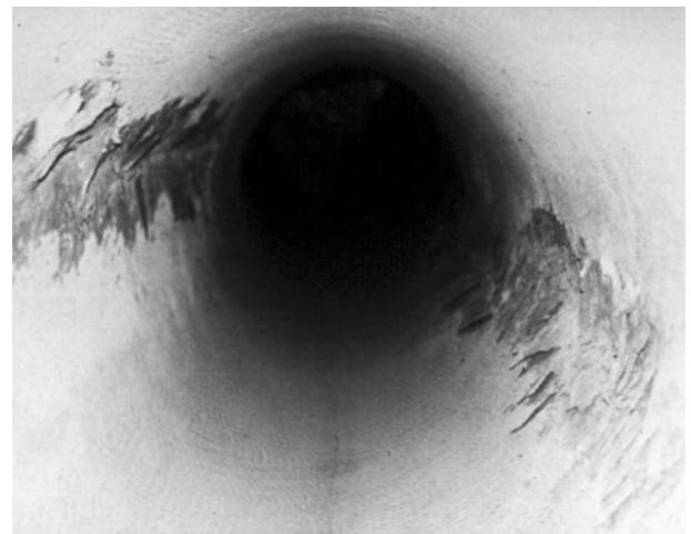
Fig. 24. Mild spalling in the sidewalls of a vertical raise bored shaft in an underground mine.
