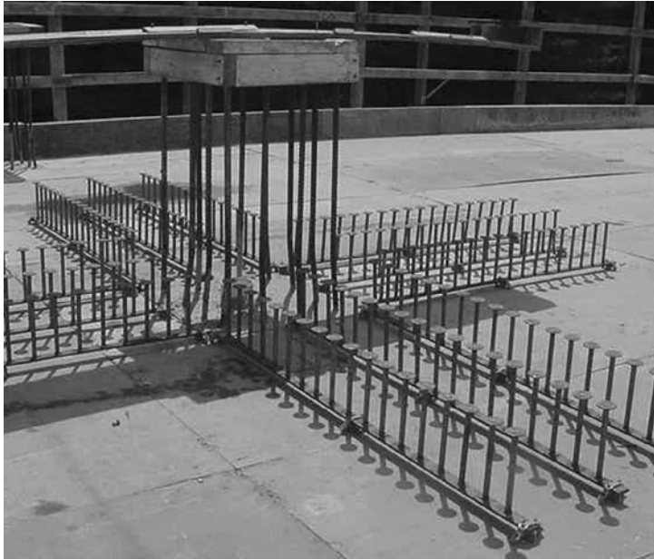
FIGURE 7.51 Headed shear reinforcement at a slab–column joint (Photo courtesy of Decon USA, Inc.).
